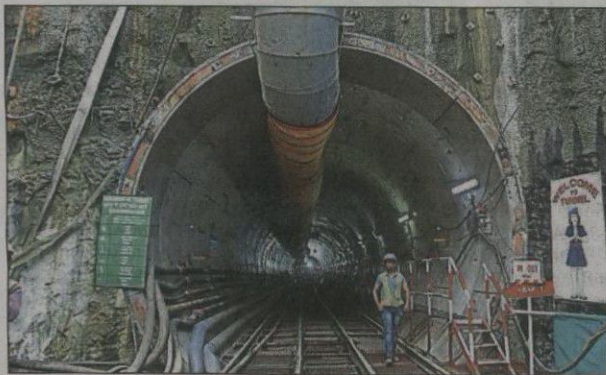
■ The tunnelling work started in November 2017 from the Naya Nagar-launching shaft in Mahim.
