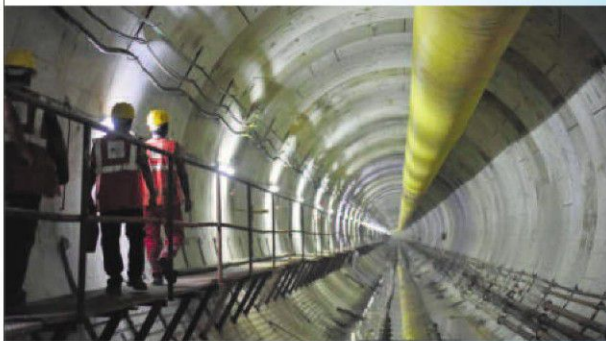
■ Workers inside the underground tunnel below Mithi River at Bandra-Kurla Complex. HT FILE
