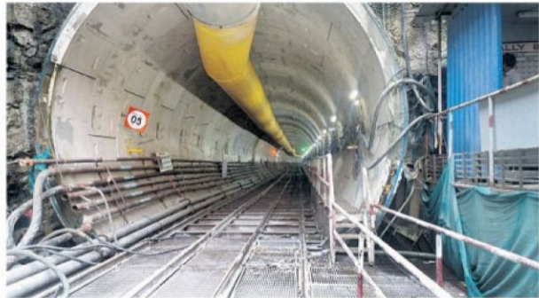
The tunnel boring machine laid down at Chhatrapati Shivaji Maharaj Terminus has now reached Girgaum
