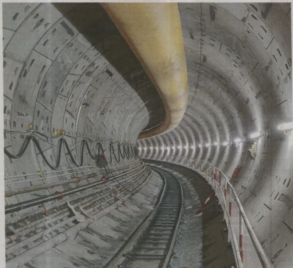
The tunnelling work of the the underground Metro work is underway in full swing.
