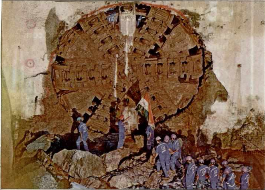
In a major landmark for the 32.5km underground Metro III corridor (Colaba-Bandra-Seepez), the breakthrough of the first tunnel-boring machine (TBM) was achieved in 259 days on Monday
