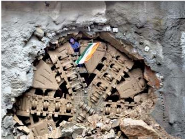
End of the journey: Tunnel Boring Machine Wainganga 2 tunneled 4.5 metres daily for 125 days. ■ SPECIAL ARRANGEMENT
