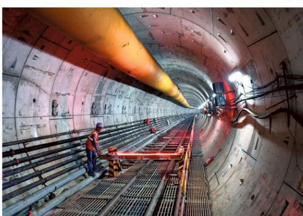
Under construction: By the end of 2019, nearly 80% of excavation and tunnelling work is scheduled to be completed. ■ FILE PHOTO
