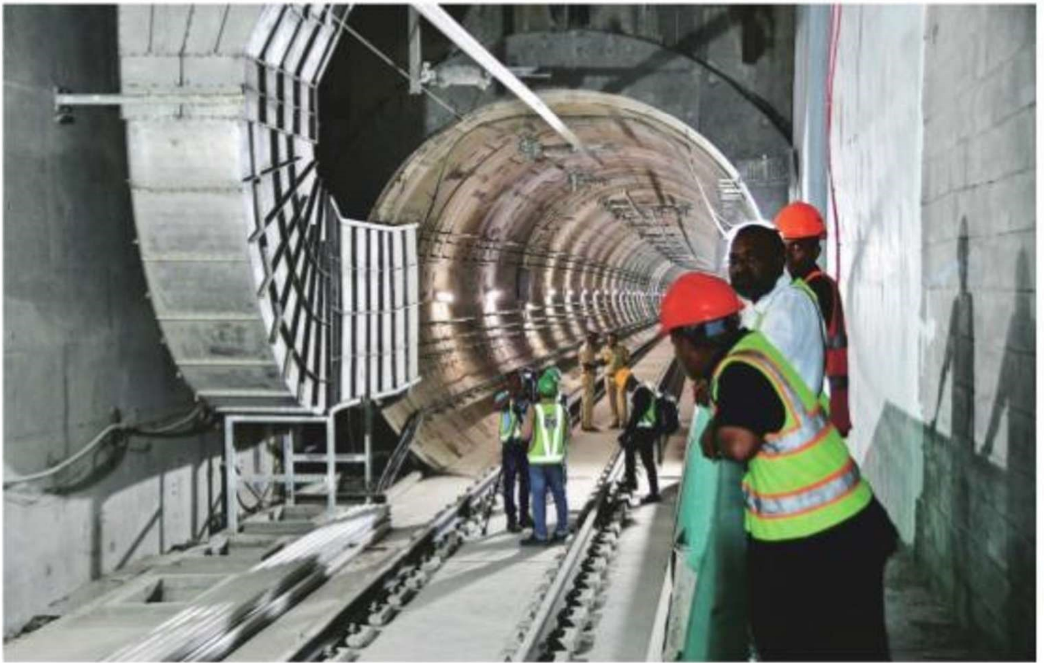
Construction work is on at the underground Metro Route 3 project at Vidhan Bhavan Metro station, Nariman Point in Mumbai, on Tuesday night. PTI
