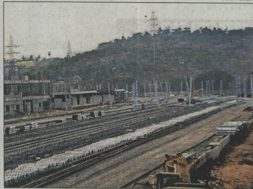
Stabling lines near Aarey Metro station. Laying of stabling line is crucial as nearly two rakes are expected to arrive every month in a few weeks
